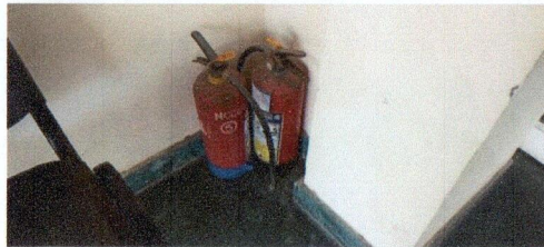
Image 5: CO 2 and ABC type fire extinguishers were provided on site.
